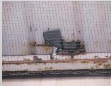
Previous repair of metal roof at rusted location
