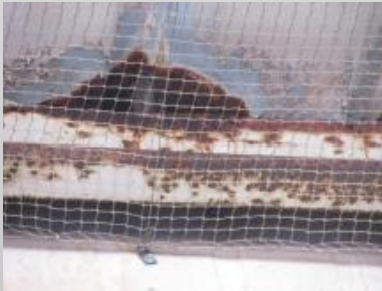
Rusted underside of roof panel
